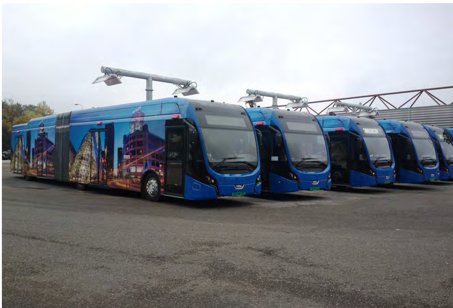
Overhead bus charging stations
